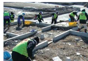
Sojitz Group employees remove debris in the disaster area.
