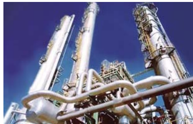
Methanol manufacturing facilities in Indonesia
