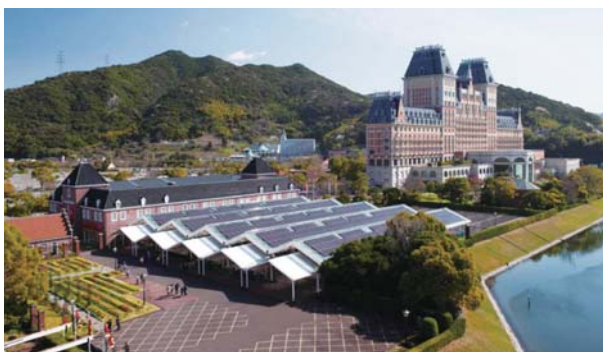
Solar panels installed at Huis Ten Bosch
